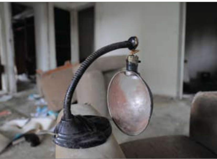
The state of things once UMAM D&R's team gained access to the building.
